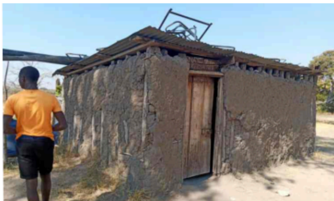
This is the structure that is currently being used as a boys' boarding facility at Kalobolelwa Secondary School
